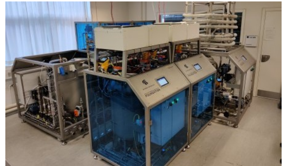
Fig. 3: Picture of the Smart Water Lab used for the tests.
